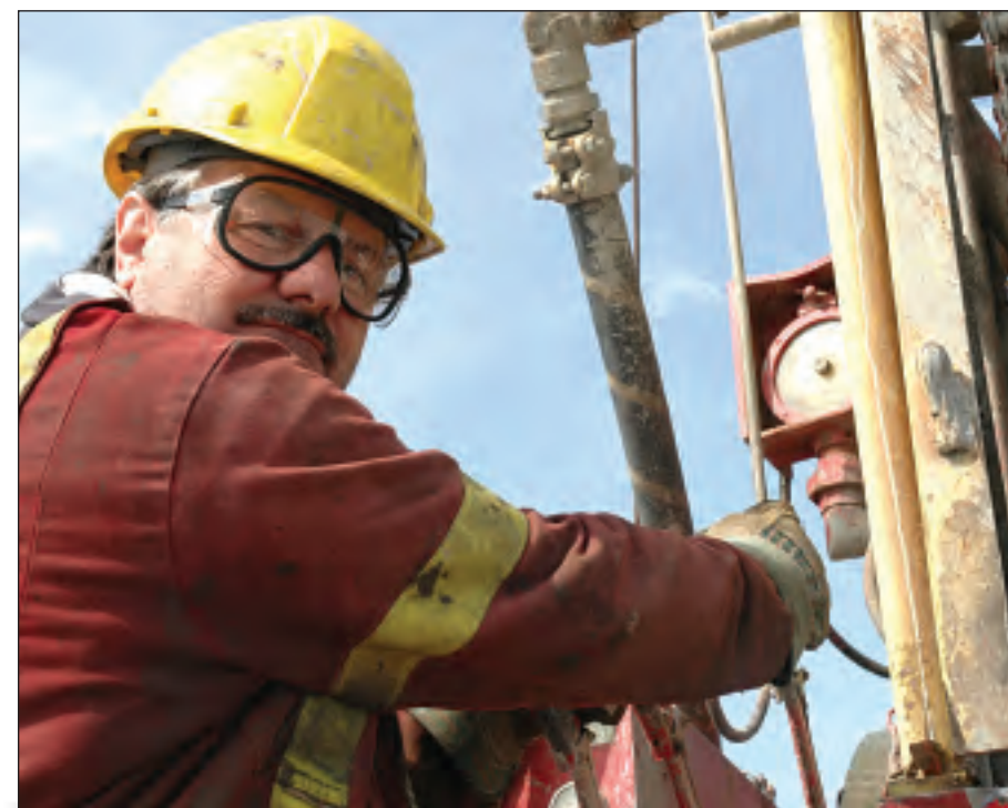
Driller Paul Marier is hard at work at the Bruce site where Phase Two of the geoscientific site characterization plan for OPG's proposed DGR, which includes the drilling of two vertical boreholes at two separate drill sites, began at the end of March.
