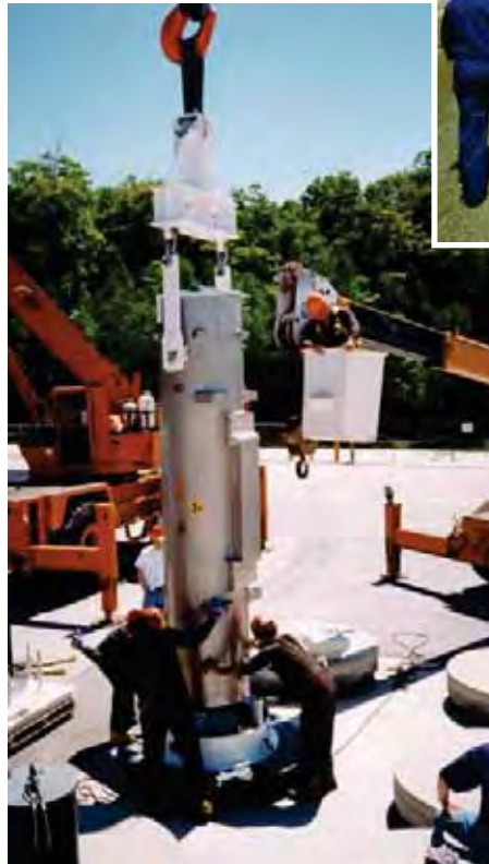
Ontario Power Generation staff carefully lower intermediate level waste into an in-ground storage container.
