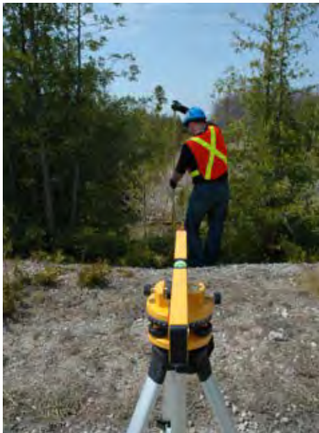
AMEC engineer Peter Nimrichter measures the elevation change across a culvert at the Bruce nuclear site as part of the mapping of the site drainage network. The information will be used in the safety assessment currently being compiled by NWMO on behalf of OPG.
