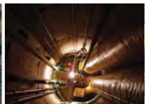
Typical shaft sinking equipment
